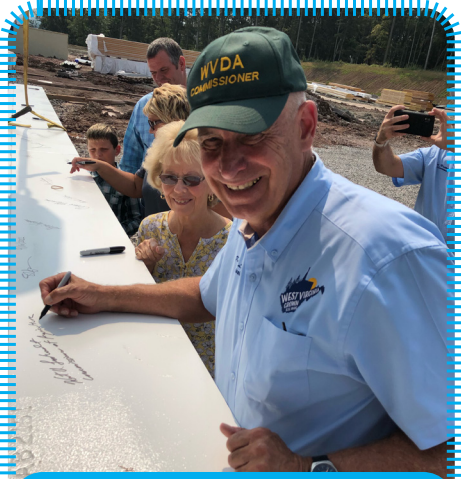
Commissioner Kent Leonhardt signs his name to the last beam put in place at the Mountaintop Beverage facility.
